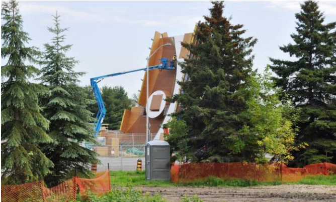
Forms for the Airport Parkway footbridge main tower, as of September 2011. Photo: Clarke/CfSC
